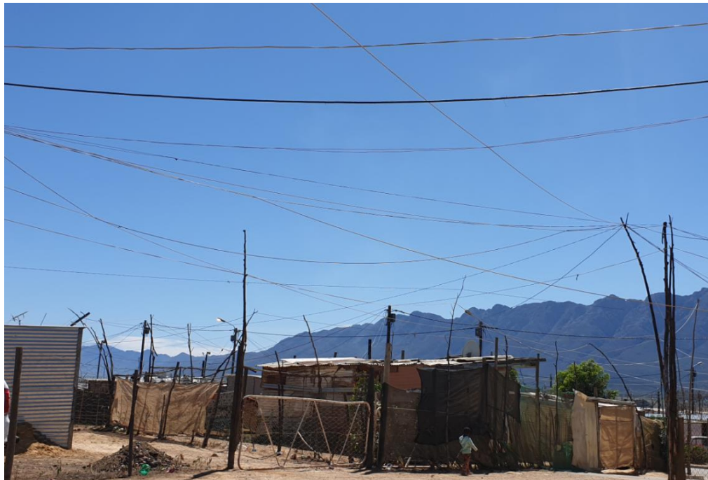
The maintenance of the electrical network remains a major challenge especially with regards to illegal connections which result in unplanned interruptions as networks becomes overloaded.
