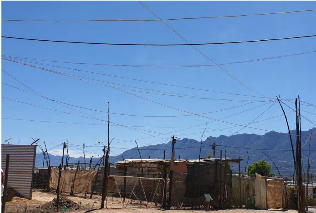
The maintenance of the electrical network remains a major challenge especially with regards to illegal connections which result in unplanned interruptions as networks becomes overloaded.
