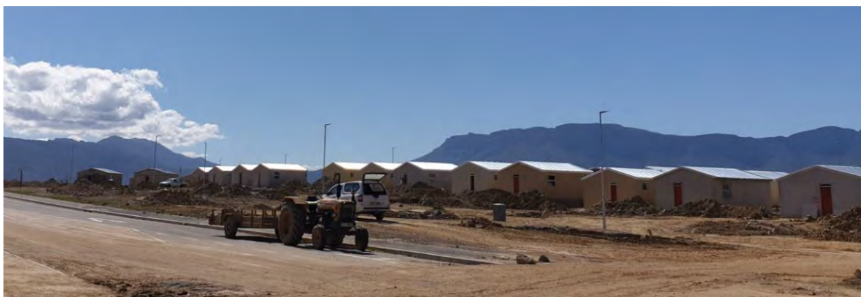
The construction of the 1 st phase of houses as Vredebes Housing development has commenced.
